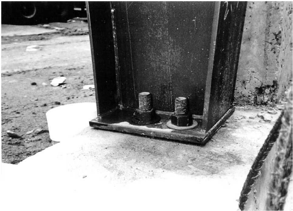
FIGURE 12.33 Closely spaced anchor bolts are acceptable for pin-base but not for fixed-base columns.
